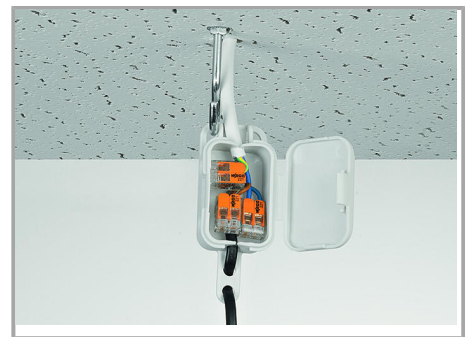
Pendant light connection in suspended ceilings
