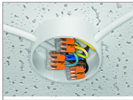
Lighting distribution in ceiling canopy
