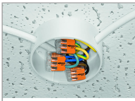
Lighting distribution in ceiling canopy
